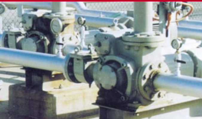
Oil Terminal load in/load out
