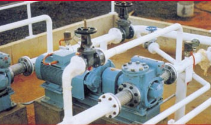
High Capacity rail tank car unloading
